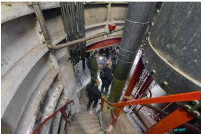
We were able to visit the southern plant room which is at a lower level close to the bottom of the lift . When the museum runs public tours which will begin later in the year this area will not be included
